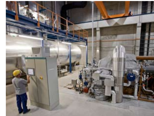
KONTROLLSTATION CONTROL STATION
